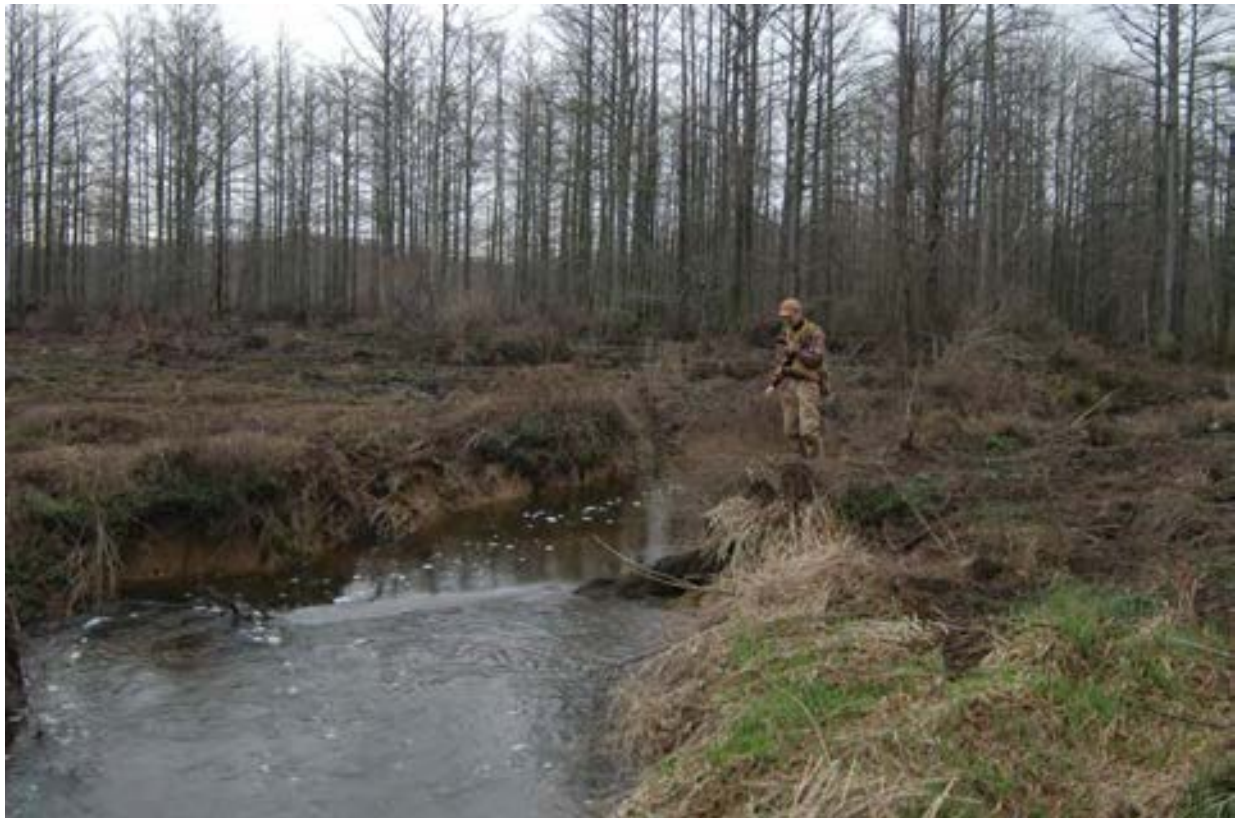
Figure 17 Looking upstream at bank erosion on Ditch 1.
