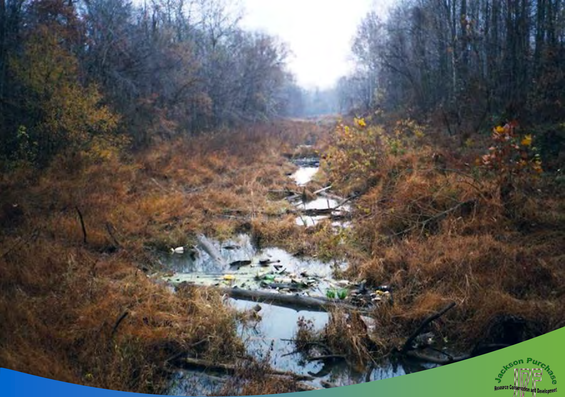
Blockage upstream of KY-307 bridge
